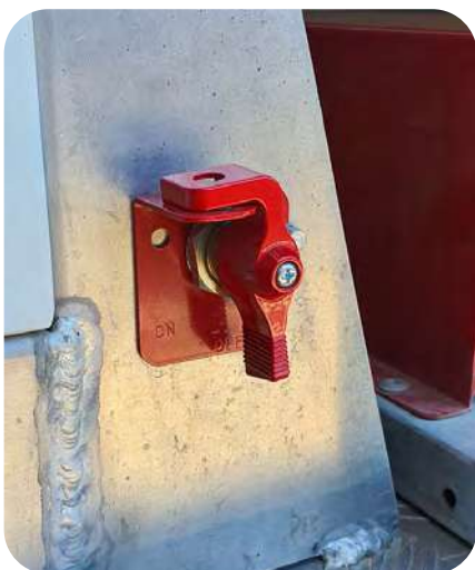
Battery Isolation Switch
